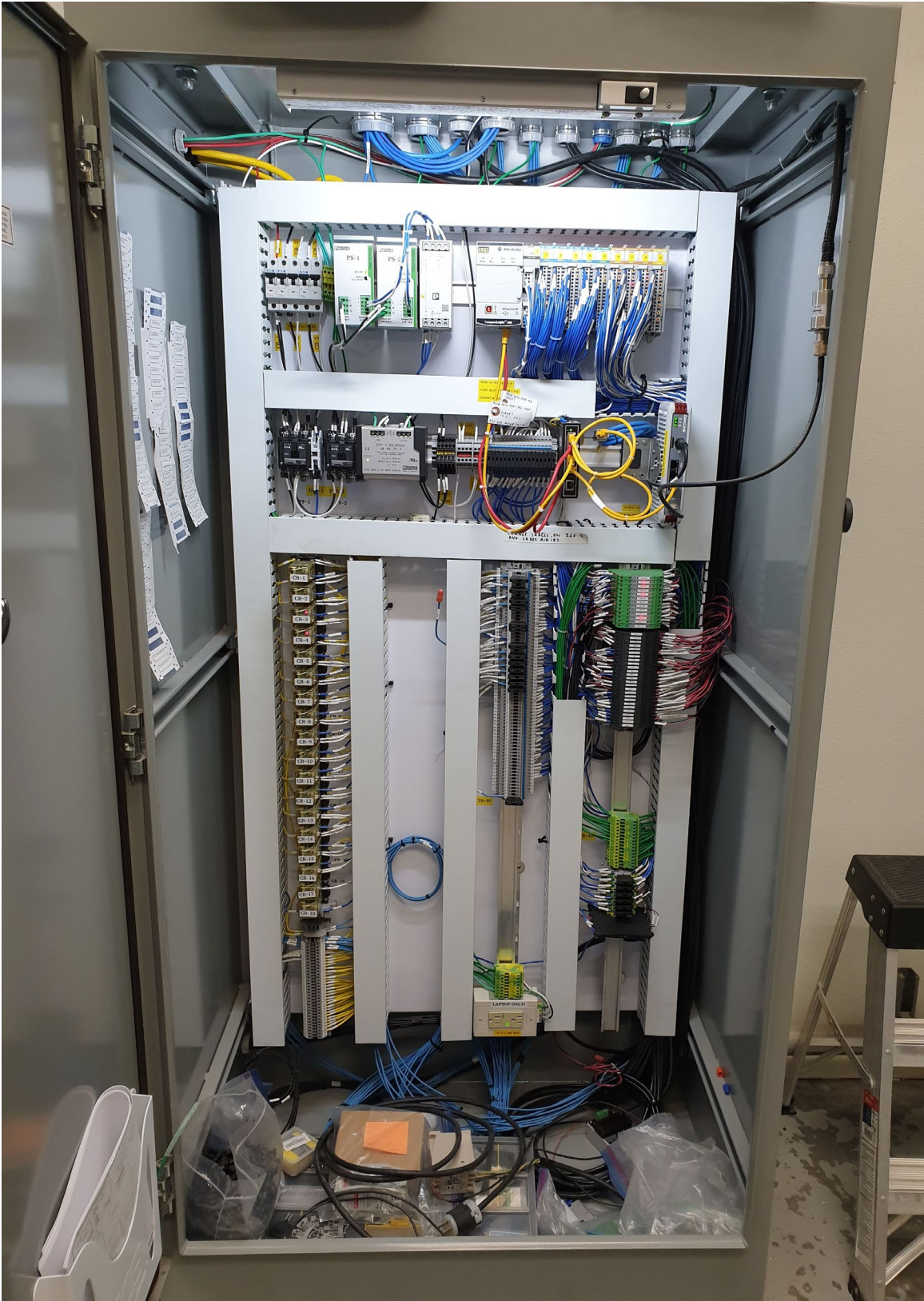
New Control Systems Engineering SCADA/PLC Control Cabinet in service at water plant main office control room.
