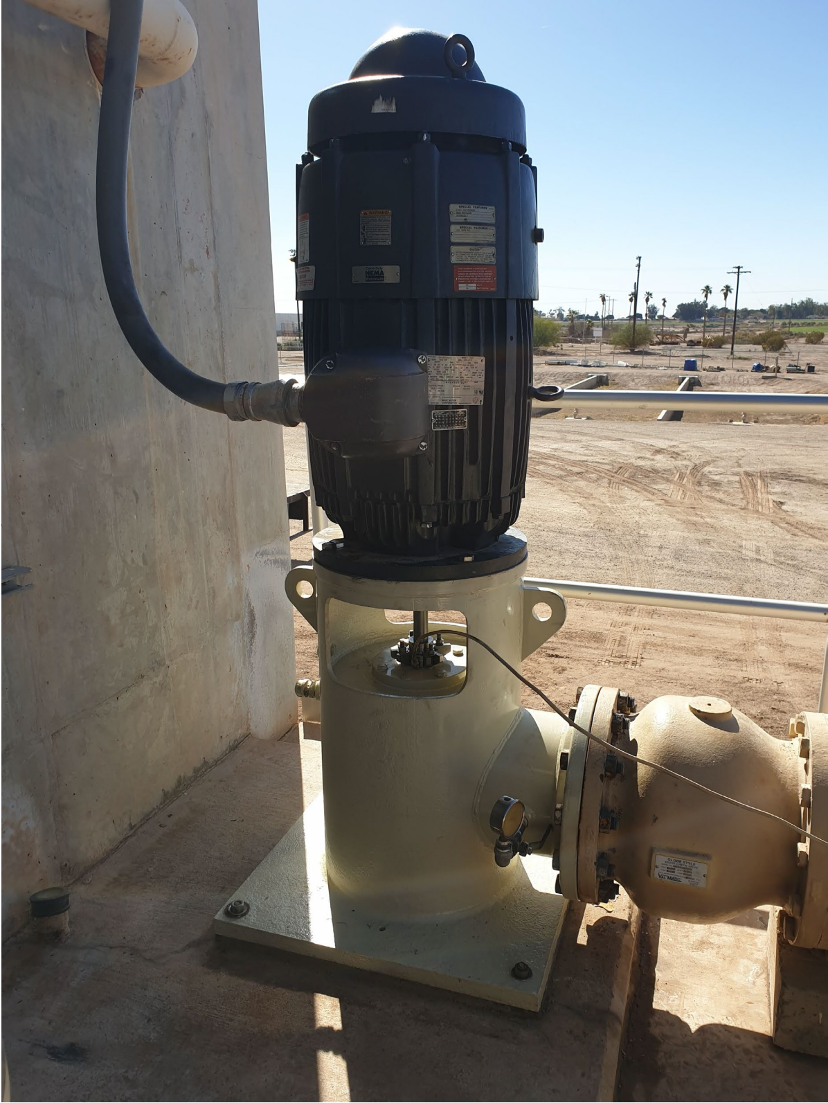
Recently rebuilt Finished Water Transfer Pump #2 with new 40 HP inverter rated motor for use with Variable Frequency Drive (VFD) controller.
