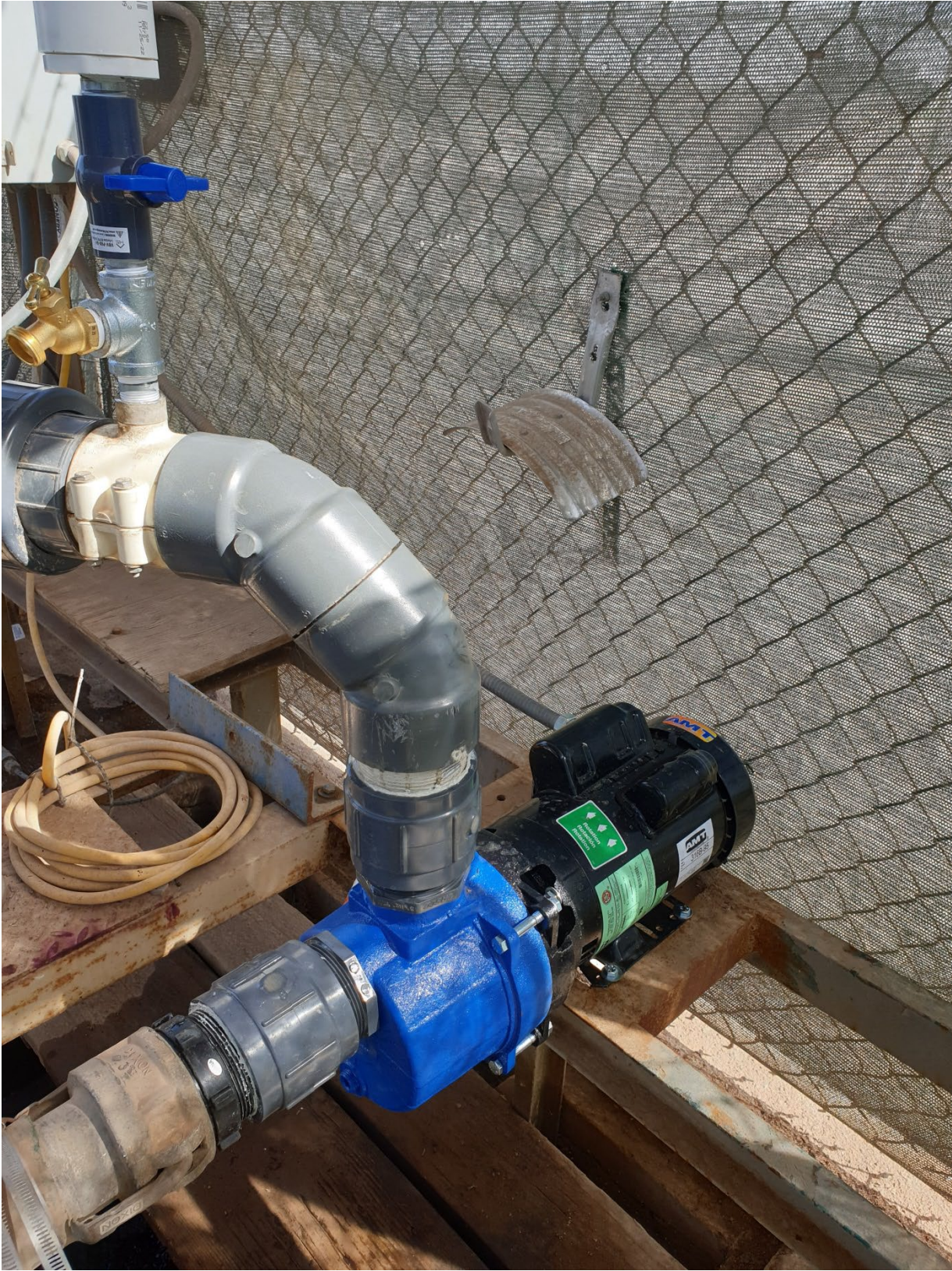
New 3" Chemical Mixing Pump installed at Raw Water Ponds Headworks for mixing of Sodium Permanganate.
