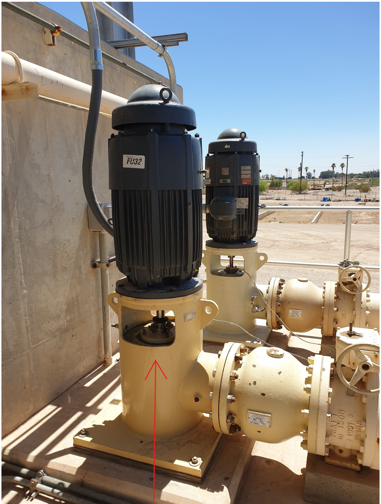
New FWTP #2 Inverter Rated 40 HP Motor
