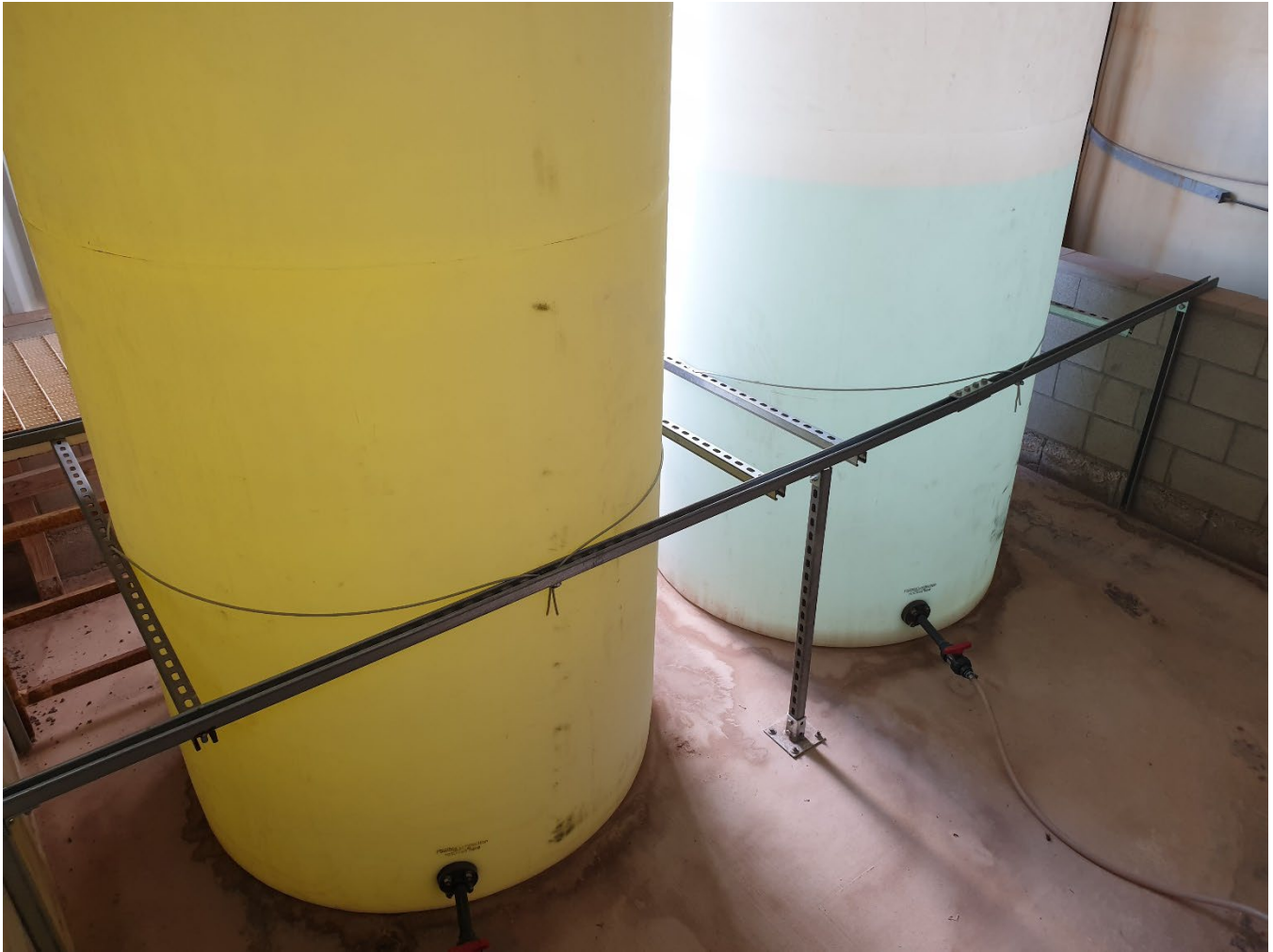
New Unistrut Channel and Cable anchoring components for spare chemical storage tanks.
