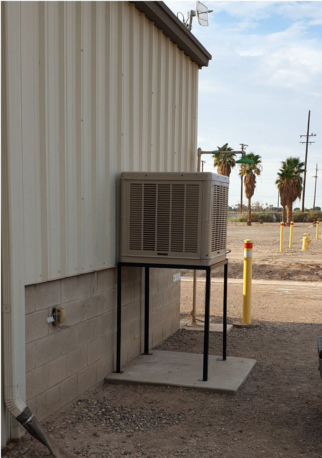
New evaporative cooling unit installed at chemical storage room at water plant.
