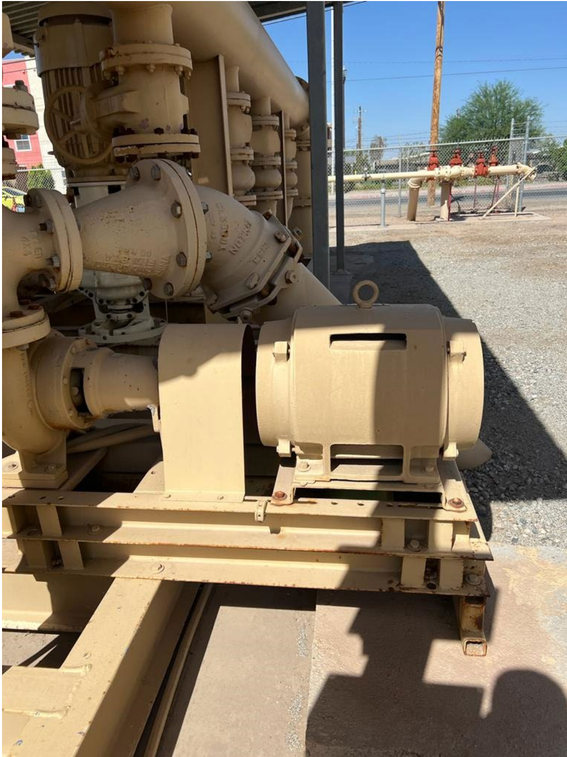
40 HP emergency standby jockey pump
