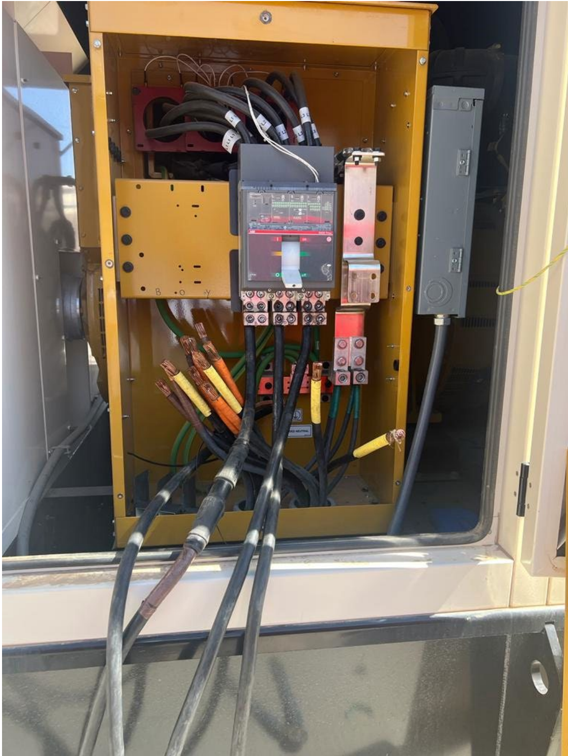
Temporary direct cable connections from water plant main generator to 40 HP emergency standby jockey pump.
