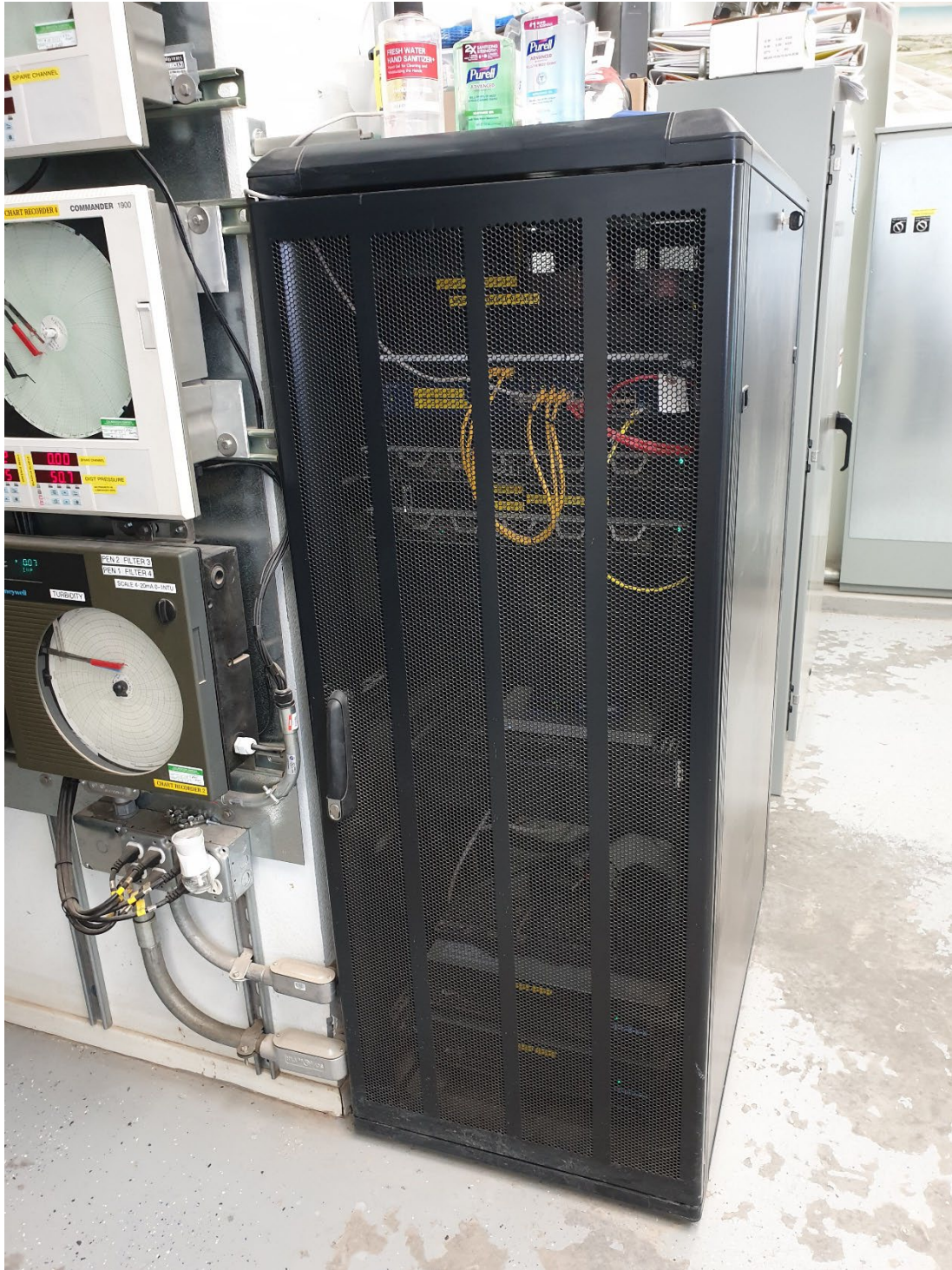
Water Plant SCADA server rack assemblies
