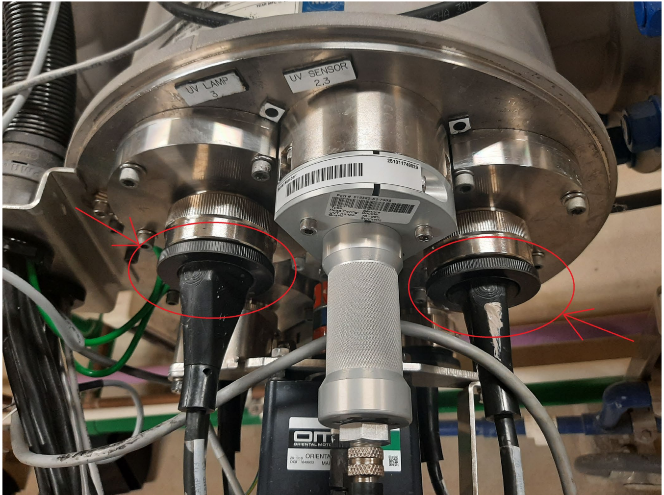
Trojan UV Sentry Train 1 sensor assemblies
