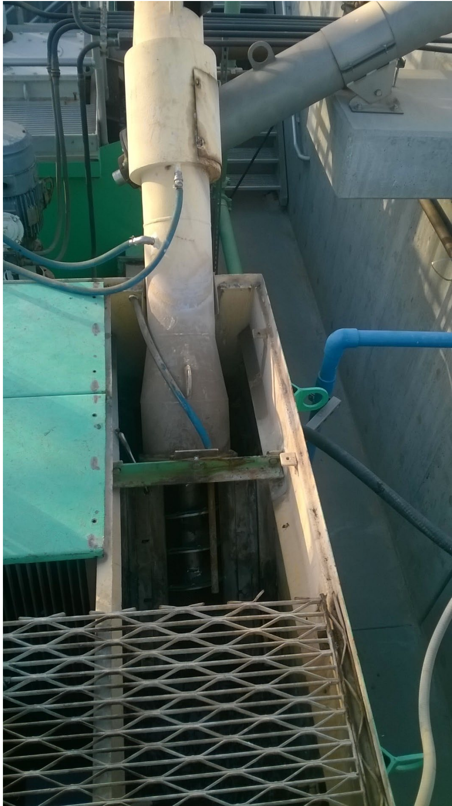
Front view of Raptor headworks auger screening unit
