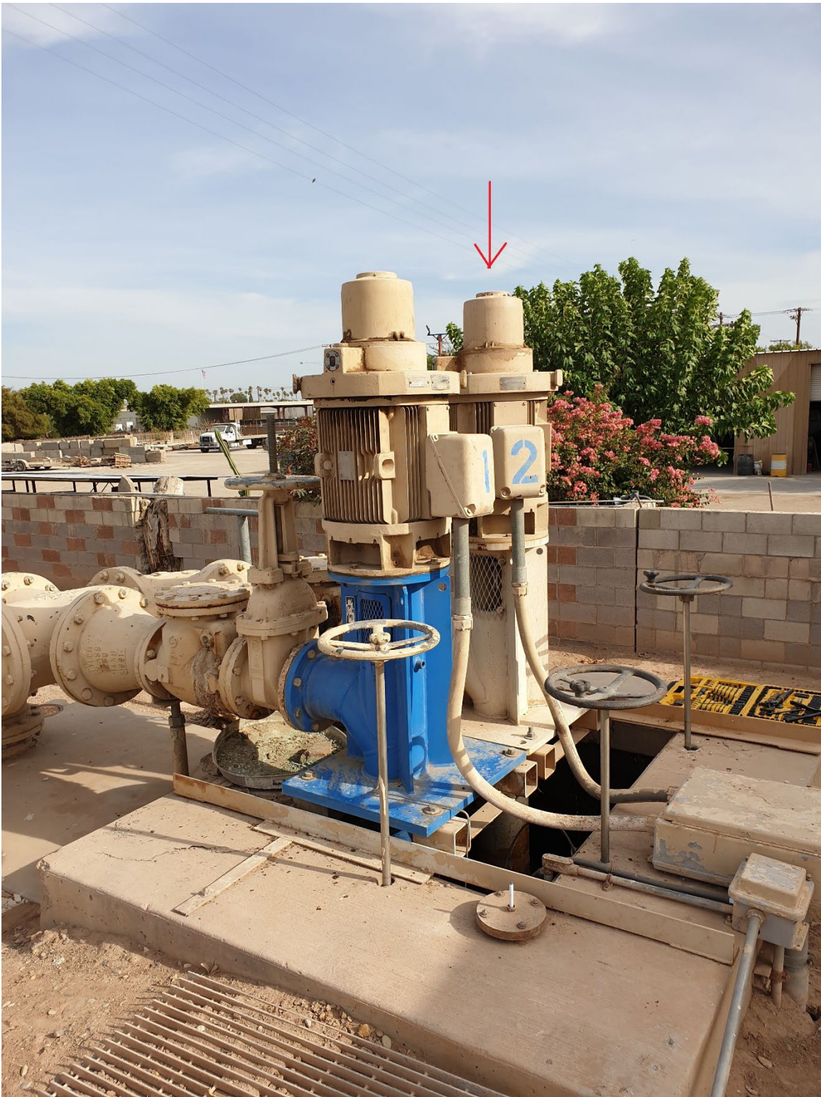
Raw Water Transfer Pump #2.
