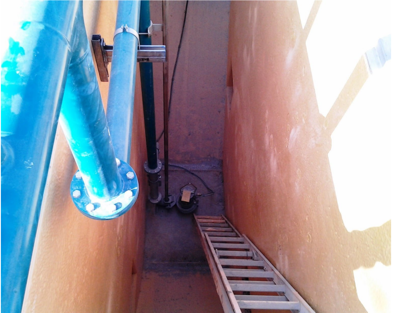
New waste activated sludge (WAS) pump installed.
