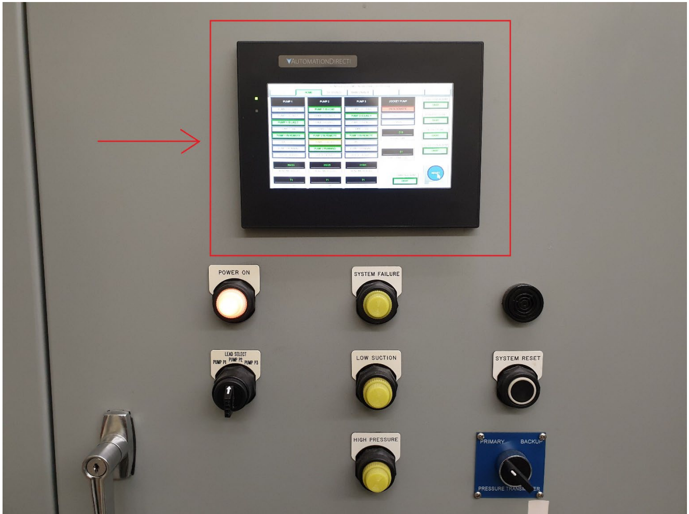
New Automation Direct Programmable Logic Controller (PLC) installed.
