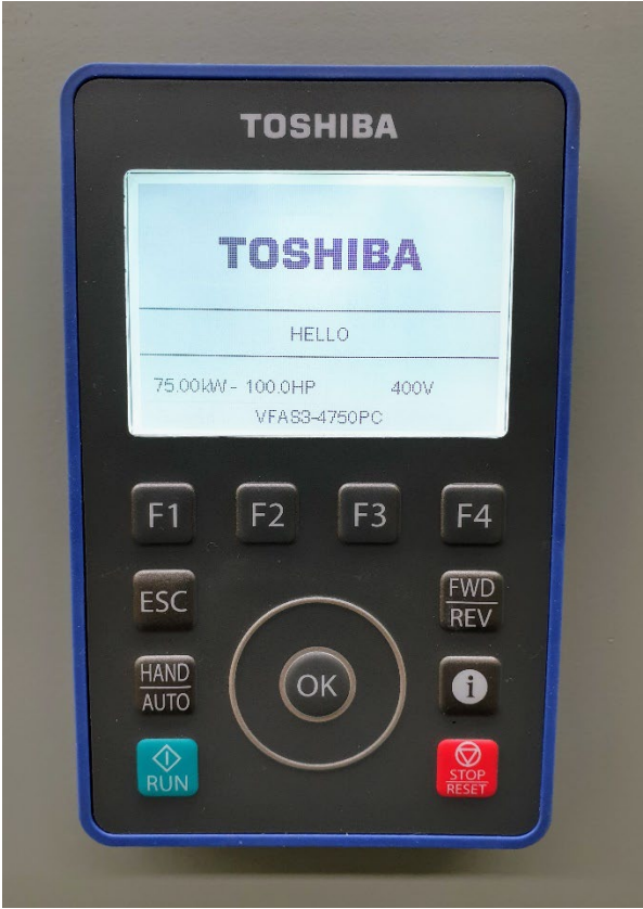
New Toshiba VFD's installed in cabinets (remote speed control pots shown on front).
