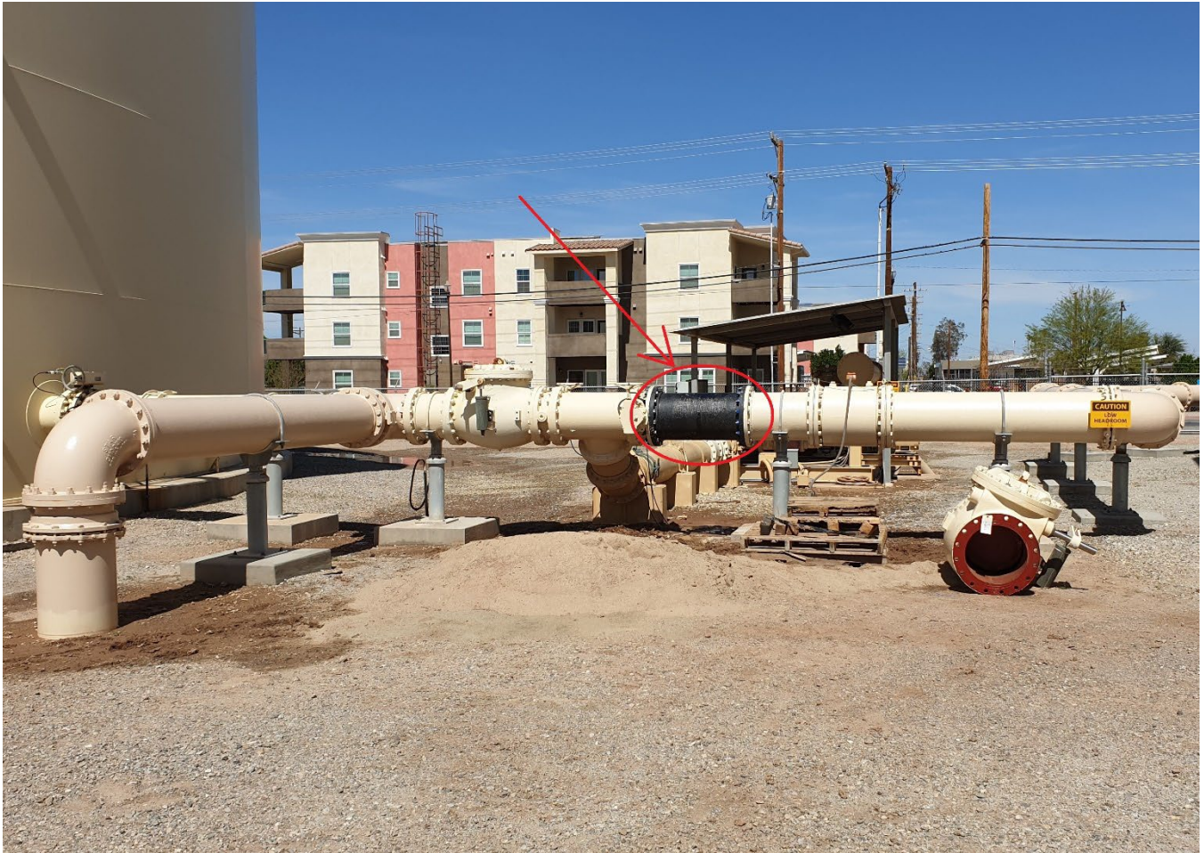
2.4 MG Tank discharge check valve replaced with an 18" cast iron spool (straight pipe).
