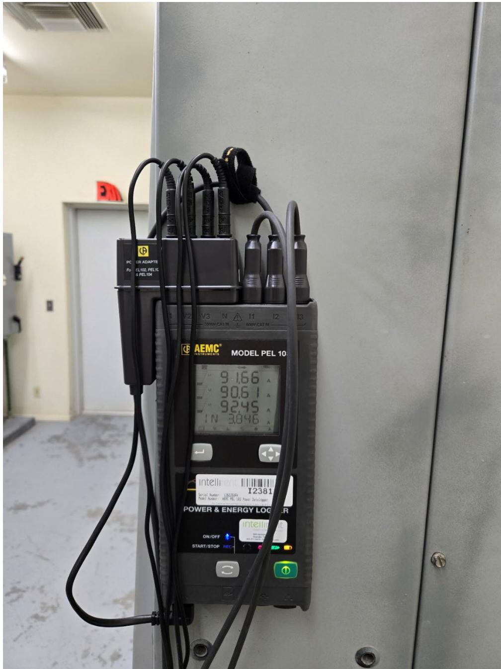
SiteLogiq continuous monitoring power usage recorder
