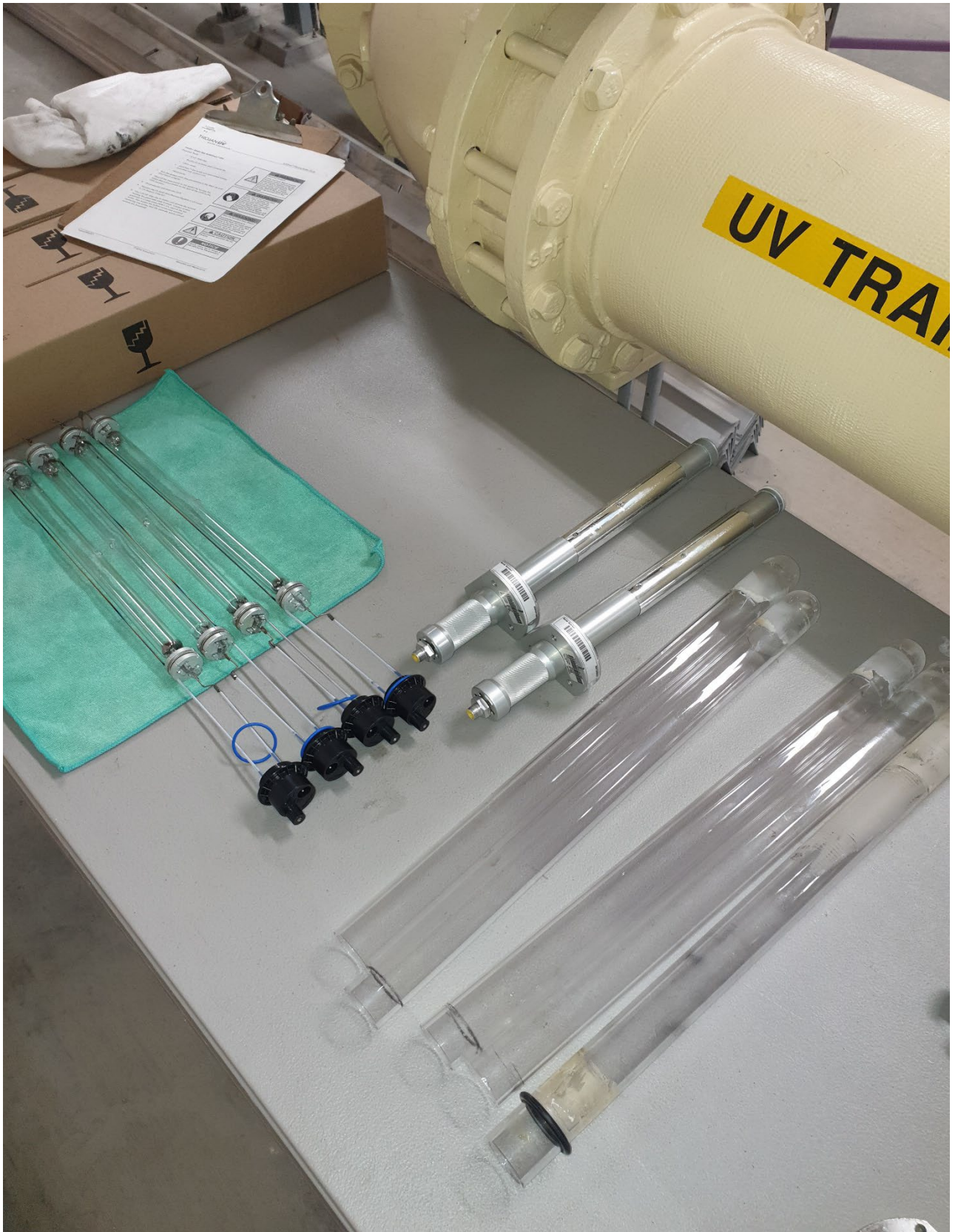
New UV lights & Sensors (Quartz sleeves before cleaning)
