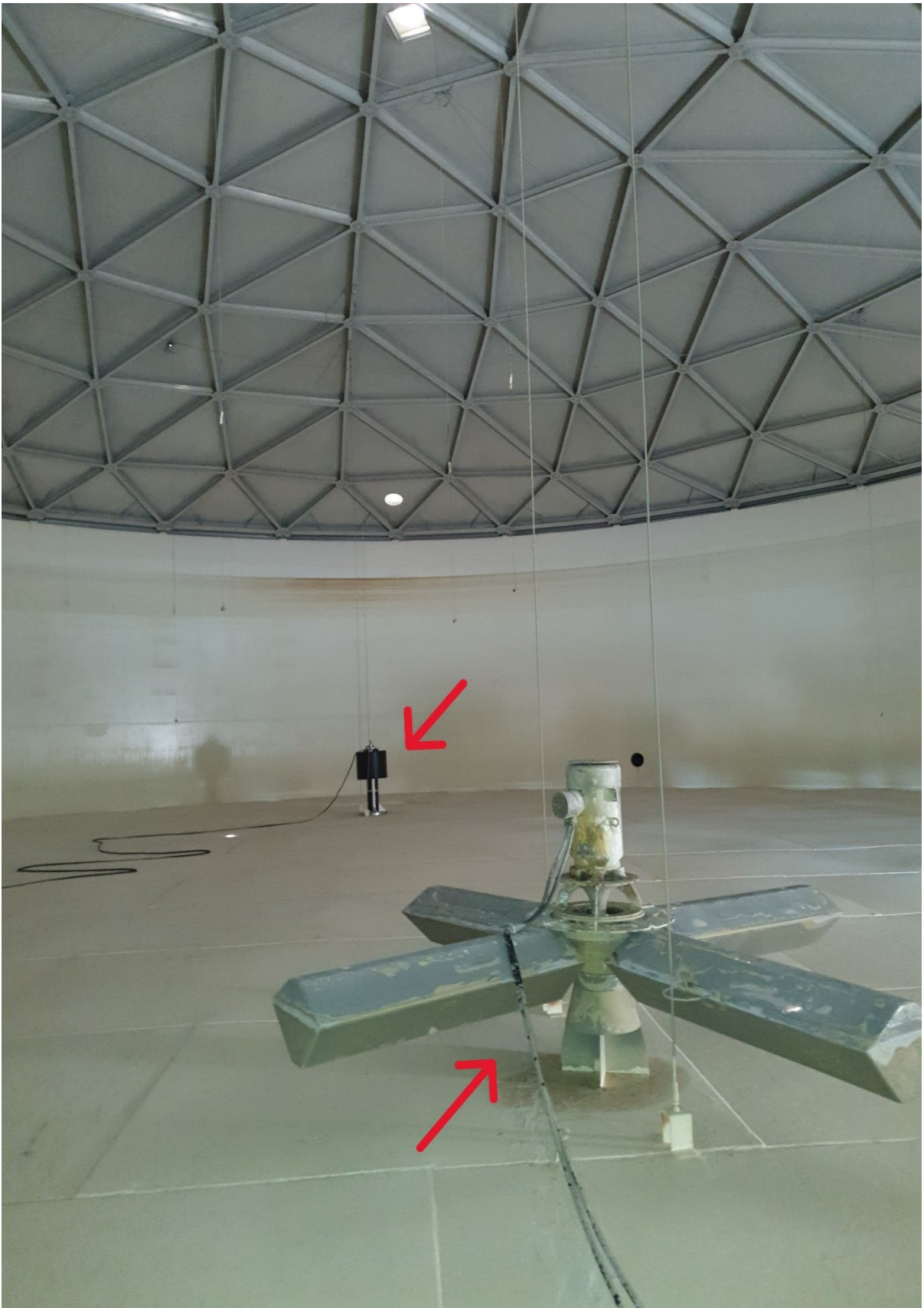
Pictures of both aerators (TTHM System) Close aerator is the old style
